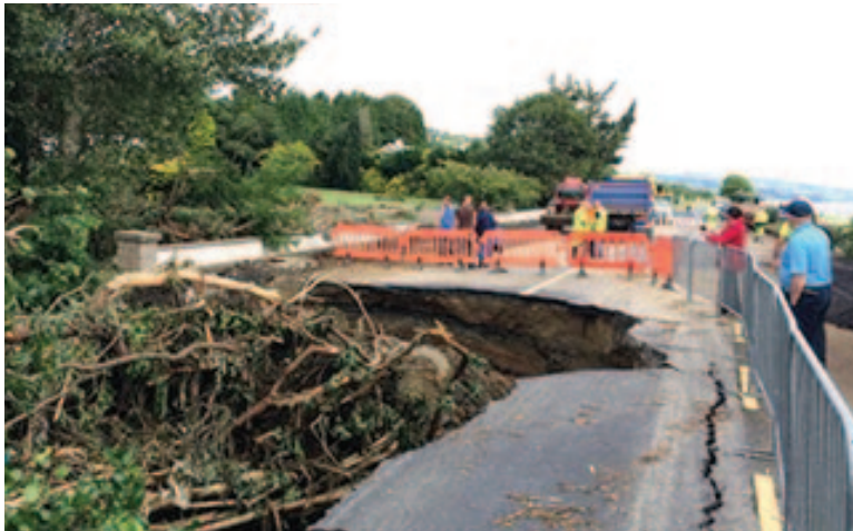
Road damage following flooding in Inishowen, Co. Donegal, 2017.
